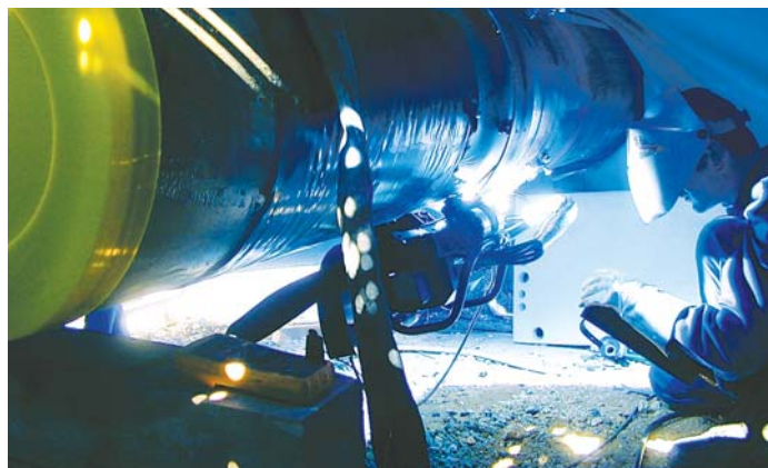
▲ FIGURE 2 A welder oversees an underground pipeline operation. Orbital welding equipment now is designed for easier transportation around a job site and is better-suited to confined spaces.
